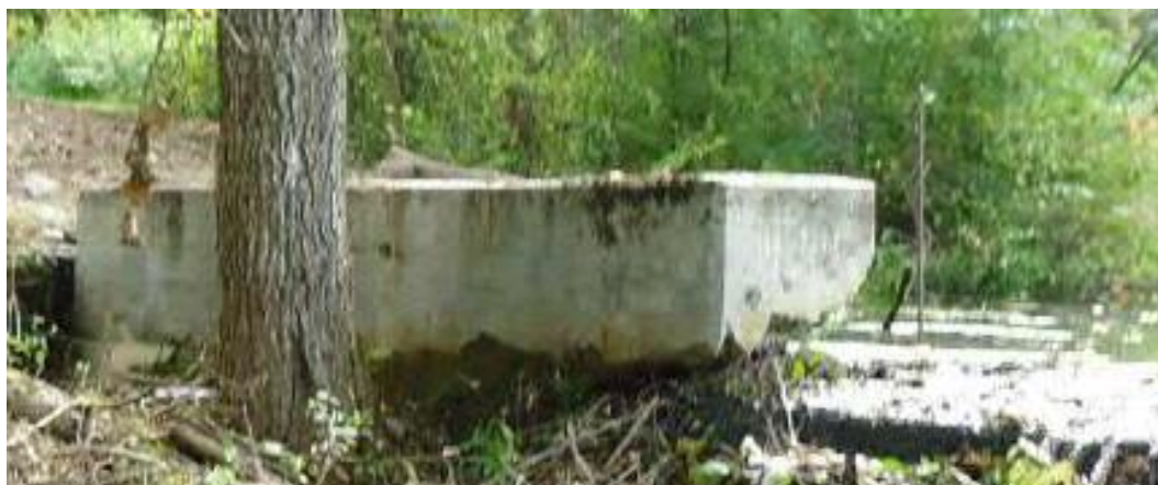
Figure 4 - Example of Undermining and Spalling of Training Wall (II) 15
