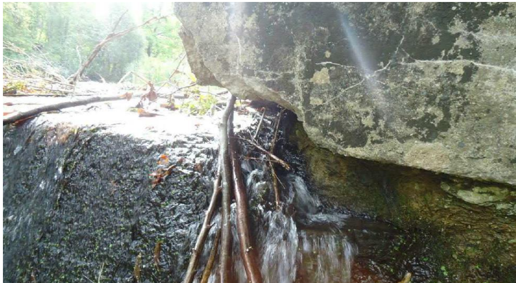
Figure 3 - Example of Undermining and Spalling of Training Wall (I) 14
