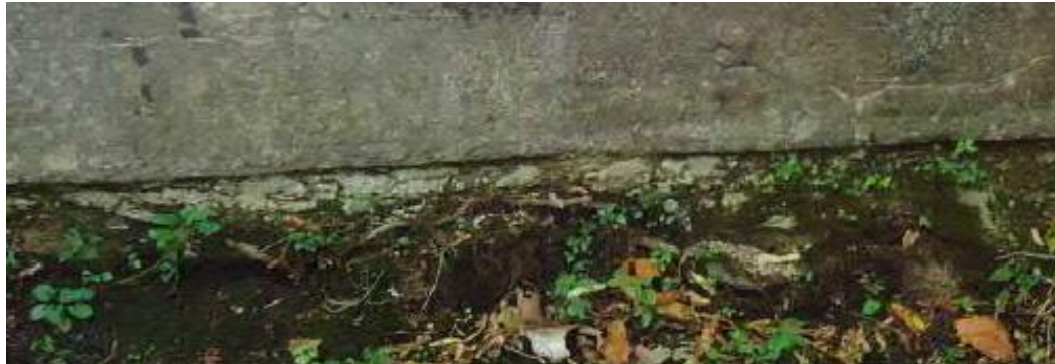
Figure 5 - Example of Crumbling and Open Joints 16
